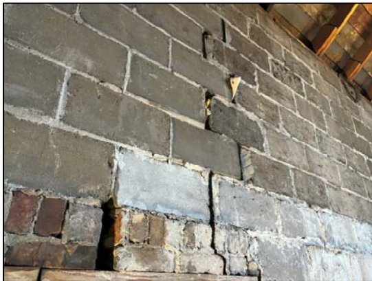
Photo 46: General view of cracked mortar and shifting blocks along the stairwell
