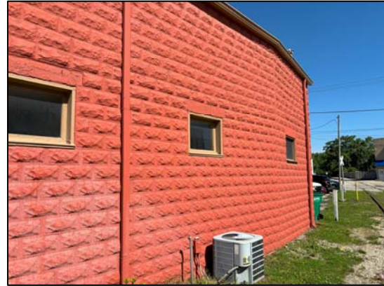
Photo 10: General view of the air conditioning unit outside
