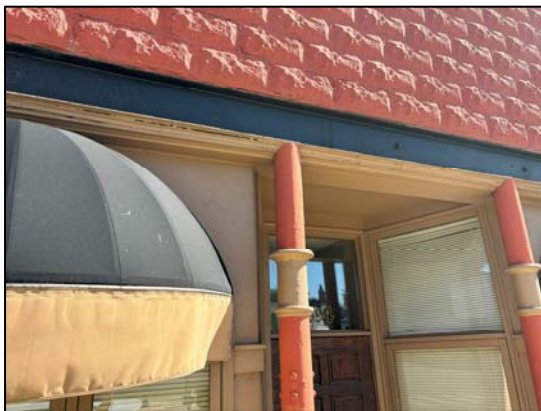
Photo 14: General view of the deteriorating sealant above the south wall windows
