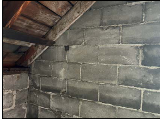
Photo 48: General view of a wall support in the northwest corner of the Building
