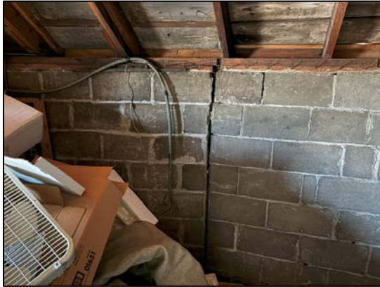
Photo 51: View of cracked and shifting concrete blocks in the northeast corner
