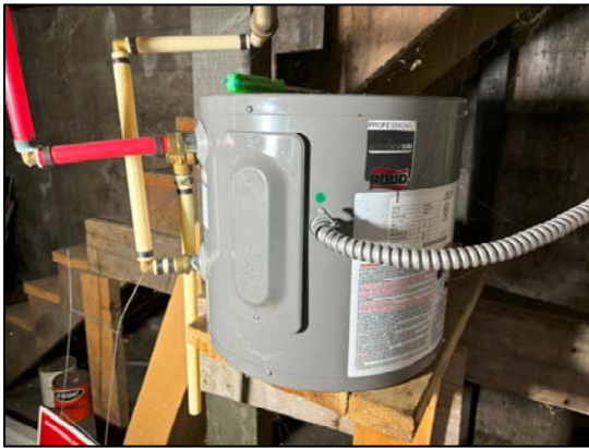
Photo 70: General view of the hot water heater along the stairwell
