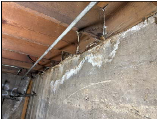
Photo 64: Another view of water-stained walls and mold growth in the southwest corner
