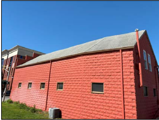
Photo 17: General view of the roof along the east side of the Building
