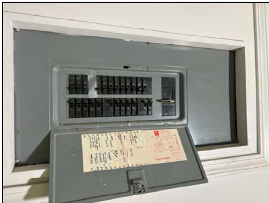
Photo 41: View of the electrical panel within the wall of the bathroom
