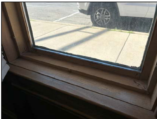
Photo 35: General view of the older wooden framed windows with water staining
