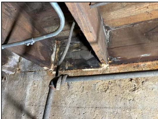
Photo 65: Another view of mold growth and deteriorating floor boards
