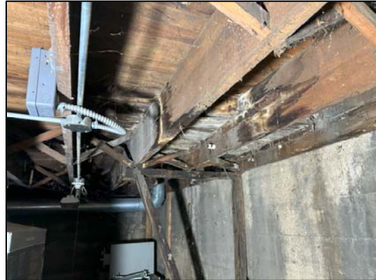
Photo 66: Another general view of water stained floor boards and mold growth
