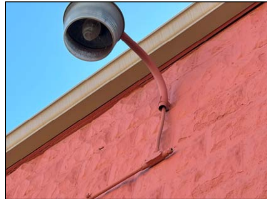
Photo 16: General view of an old light fixture along the west wall
