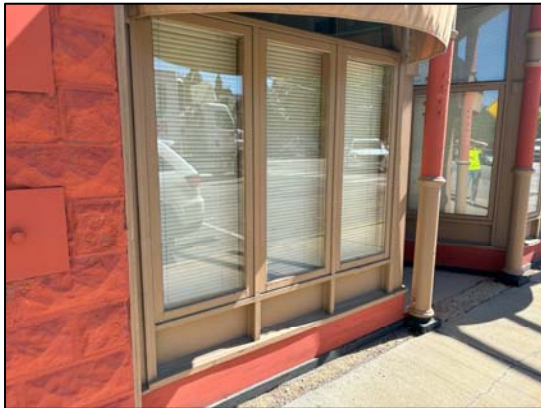
Photo 13: General view of the older wooden framed windows along the south wall
