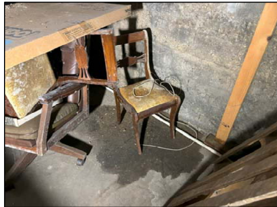
Photo 67: General view of the water stained floor slab
