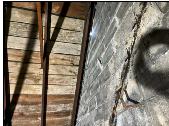
Photo 55: View of an improperly sealed roof
