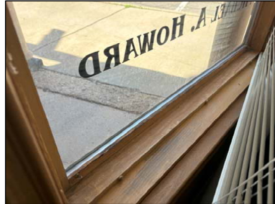
Photo 36: Another view of the older wooden stained windows with water staining
