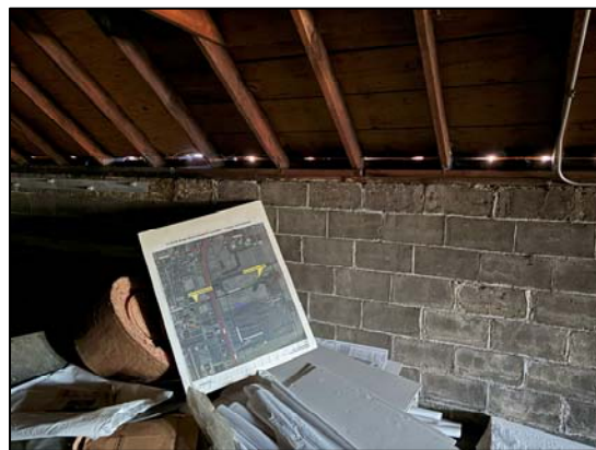
Photo 22: View of improperly sealed soffit along the roof and wall line
