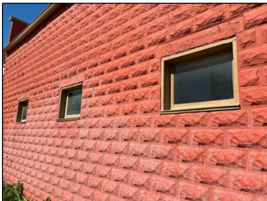
Photo 9: General view of the older wooden framed windows along the east wall
