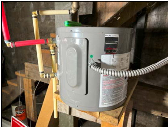
Photo 70: General view of the hot water heater along the stairwell
