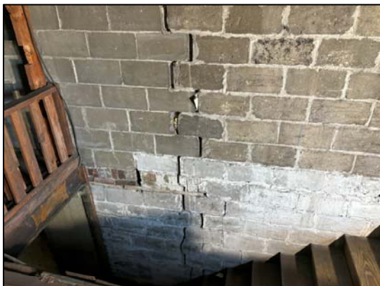
Photo 47: Another view of cracked mortar and shifting blocks along the stairwell
