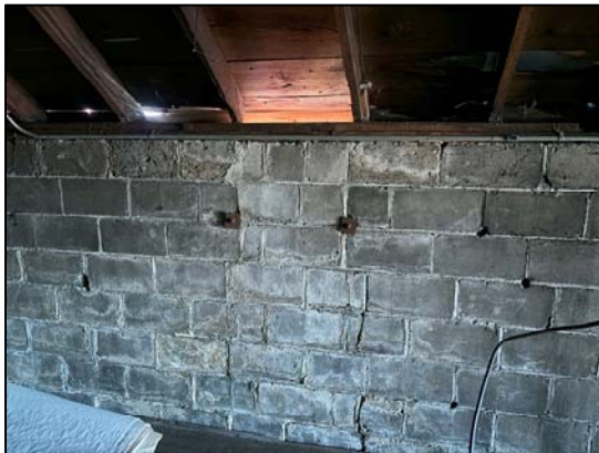
Photo 24: Another view of improperly sealed soffit along the roof and wall line
