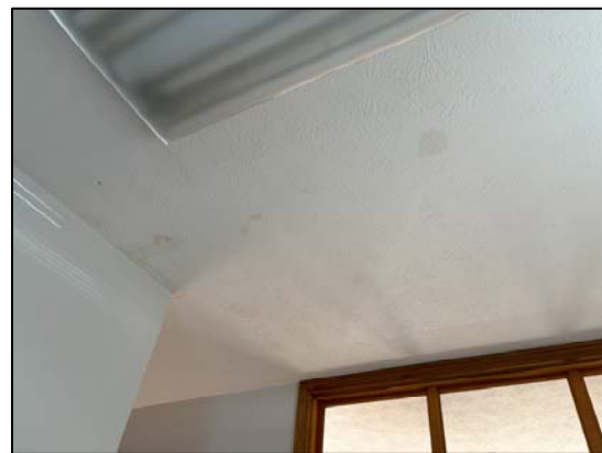
Photo 32: View of the water stained ceiling in the south section of the first floor
