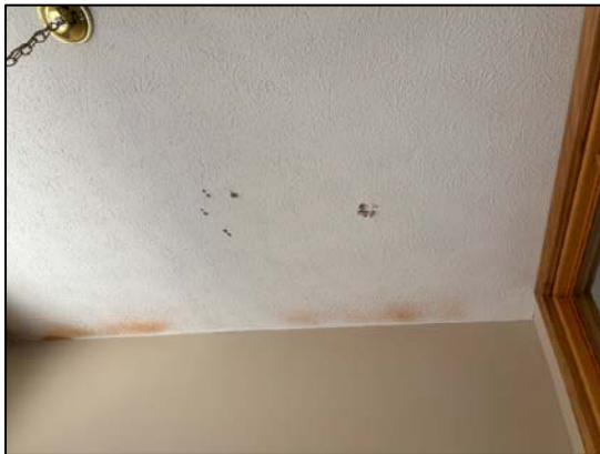
Photo 34: View of damaged drywall ceiling in the front lobby
