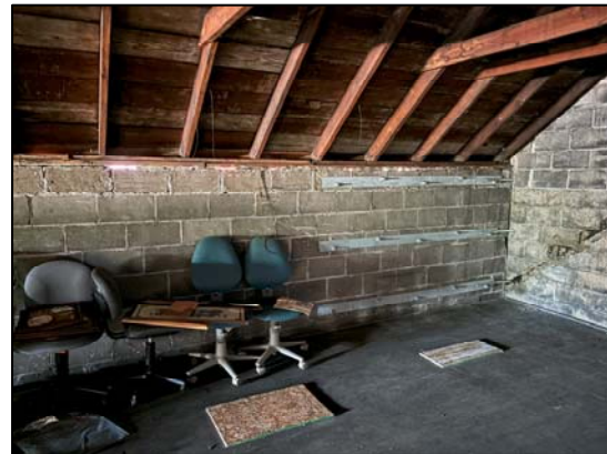
Photo 26: Another view of the improperly sealed boards to the top of the concrete block wall
