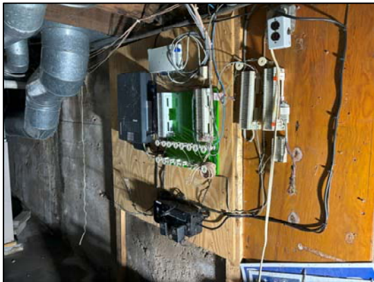
Photo 58: General view of the telecoms board in the basement
