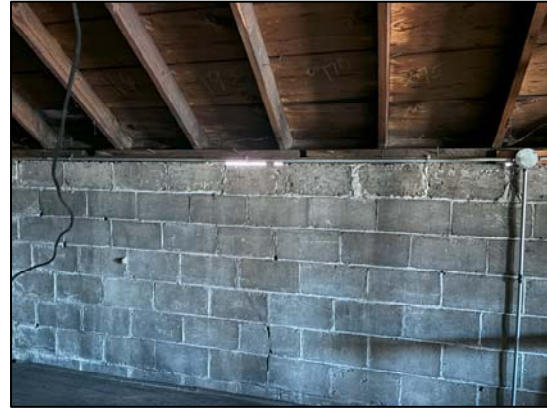
Photo 25: View of the improperly sealed boards to the top of the concrete block wall
