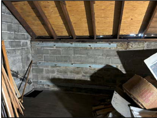
Photo 23: Another view of improperly sealed soffit along the roof and wall line
