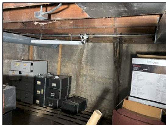
Photo 68: General view of the south wall and water stains along it
