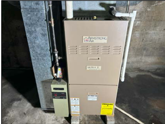
Photo 63: General view of the HVAC system within the basement
