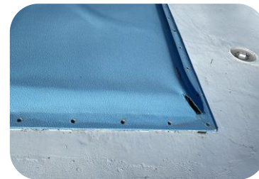
The landing pad for the small waterslide has rips in it.
