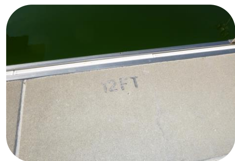
Dive pool depth markers need to be repainted or replaced with tile markers.
