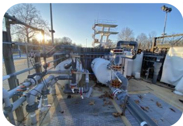
The recirculation system is exposed to the outdoor elements which decreases its expected lifespan.
