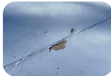
Areas of bare concrete were observed where the pool paint has delaminated.
