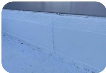
Vertical and horizontal cracking exists in the recreation pool walls.
