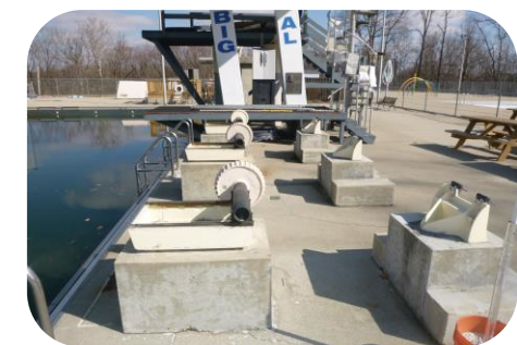
Several of the 1-meter diving boards do not have side rails installed.
