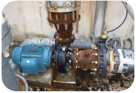
Code requirement for turnover rate which is 6 hours (main pool – 6.15 hours, dive pool – 9.7 hours) is not met with either pool.
