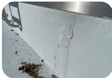
Gaps exist beneath the pool's stainless-steel gutters where it connects to the concrete wall.
