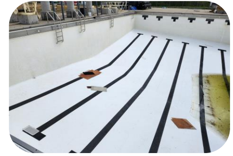
A pool liner/membrane was installed in both pools in 2012 due to significant water loss that was occurring in the main pool which is typically due to failures in the pool structure and/or the original cast iron piping.
