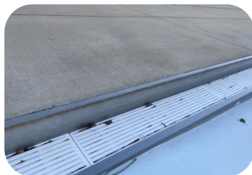
The stainless-steel perimeter overflow system had areas of corrosion.
