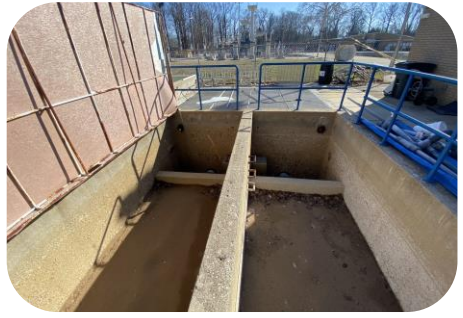
The pools' filtration is an open-air gravity sand filtration should be replaced with either high-rate sand filtration or regenerative media filtration.
