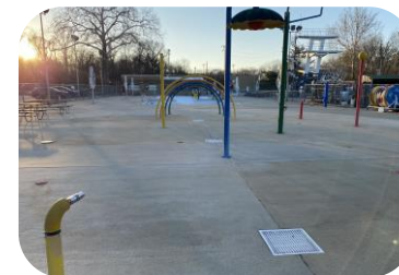
Several of the spray elements are no longer functional.
