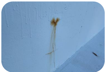
Corrosion exists on the side walls of the recreation pool where it appears the chlorinated water has penetrated the concrete shell and reached the embedded rebar.
