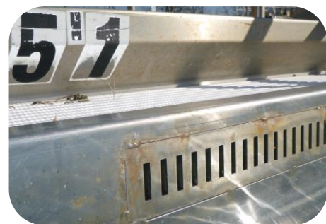
Corrosion was observed on the stainless-steel perimeter overflow system.
