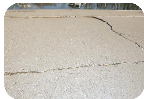
Several areas of the pool deck are in poor condition and need to be replaced.
