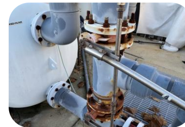
Corrosion exists on components of the recirculation system including the pipe connections, pipe supports, pool pumps and motors, and on the high-rate sand filters.
