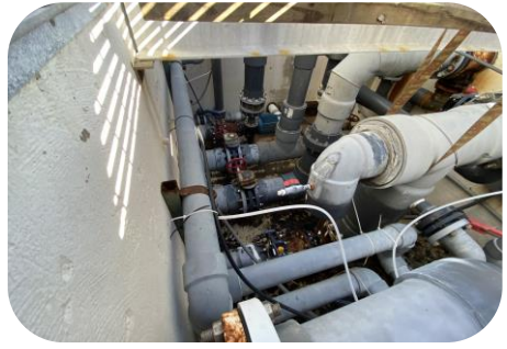
Mechanical system is exposed to the outdoor elements which decreases its expected lifespan.
