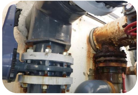
Significant corrosion on piping connections and pipe supports, and the waterslides' pump and strainer basket show similar signs of corrosion.
