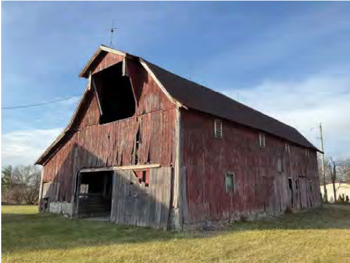
19. Looking NW at gambrel barn on Wiseman Farm (IHSSI #057-541-40032, Contributing); Lochmueller recommended rating of Notable/NRHP-eligible
