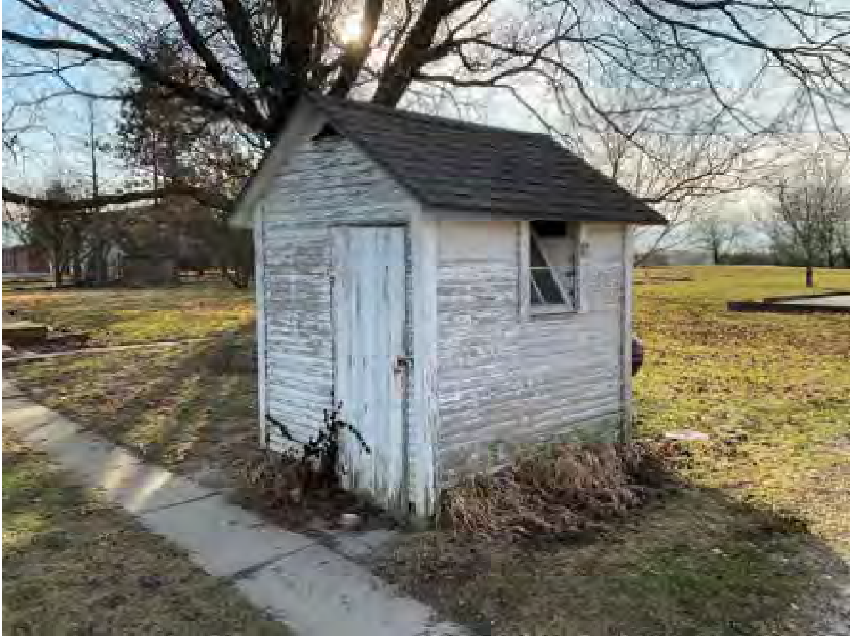
13. Looking SW at well house on Wiseman Farm (IHSSI #057-541-40032, Contributing); Lochmueller recommended rating of Notable/NRHP-eligible
