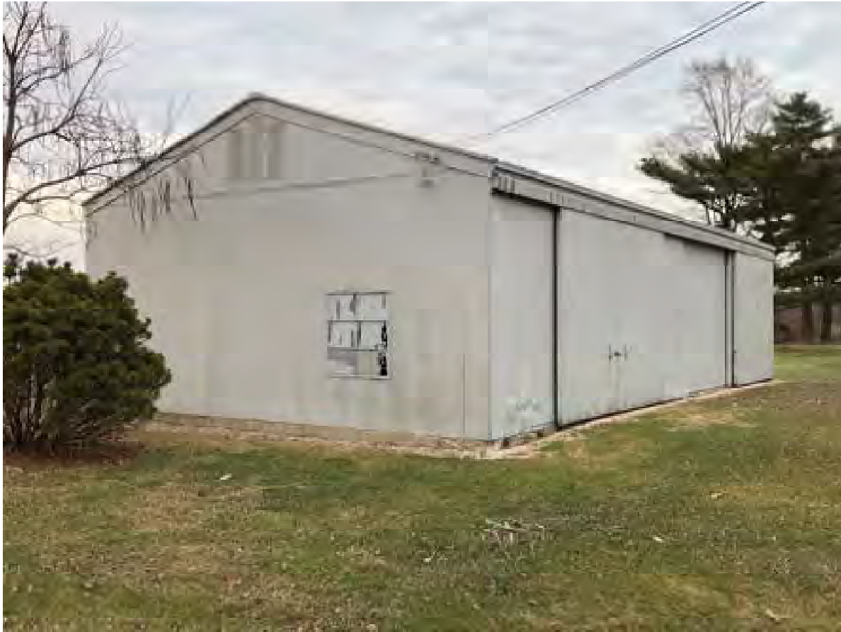
51. Looking NE at c. 1950 pole barn on Hair-Whitaker Farm (Lochmueller #4, Notable, NRHP-eligible)
