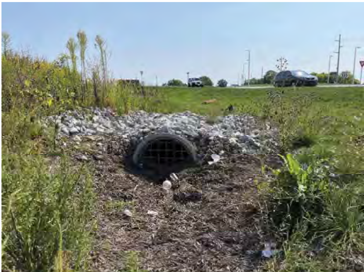
132. Looking south at culvert along east side of Olio Road north of 146 th Street within Wetland 4- 9/14/22
