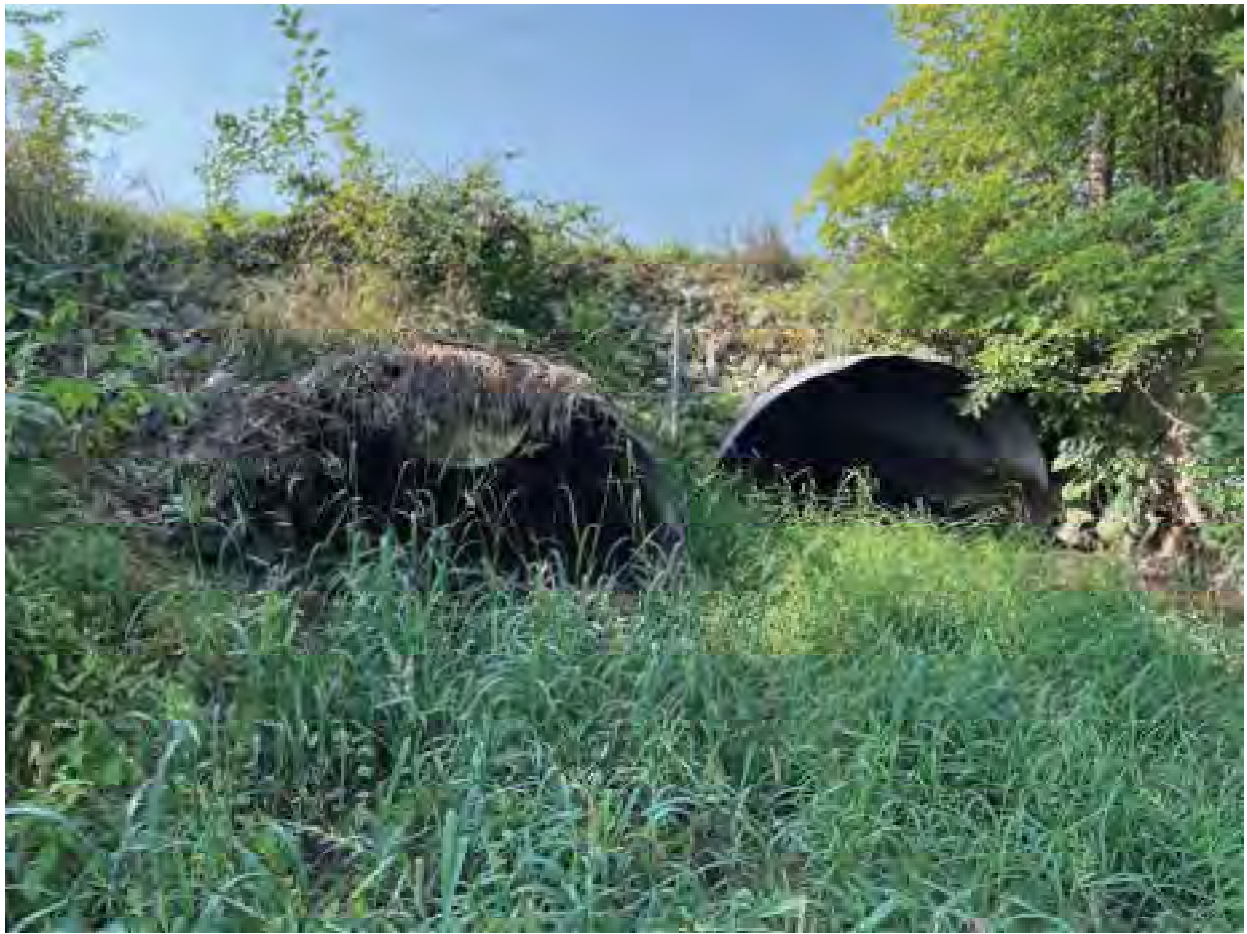
29. Looking southwest at dual culverts under 156 th Street downstream along Sand Creek- 9/14/22
