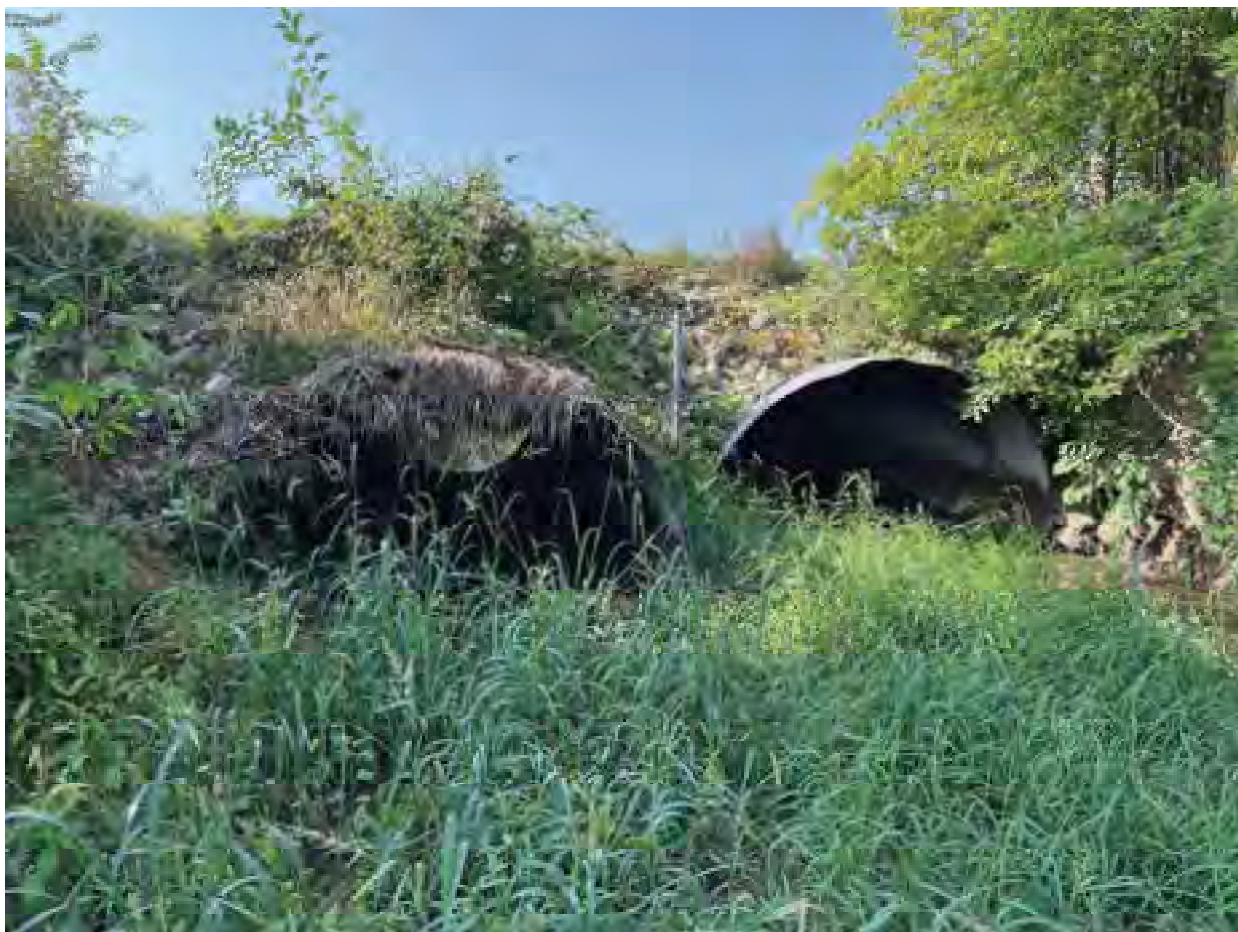
10. Looking southwest at dual culverts (Bridge #29-00277) under 156 th Street downstream along Sand Creek
